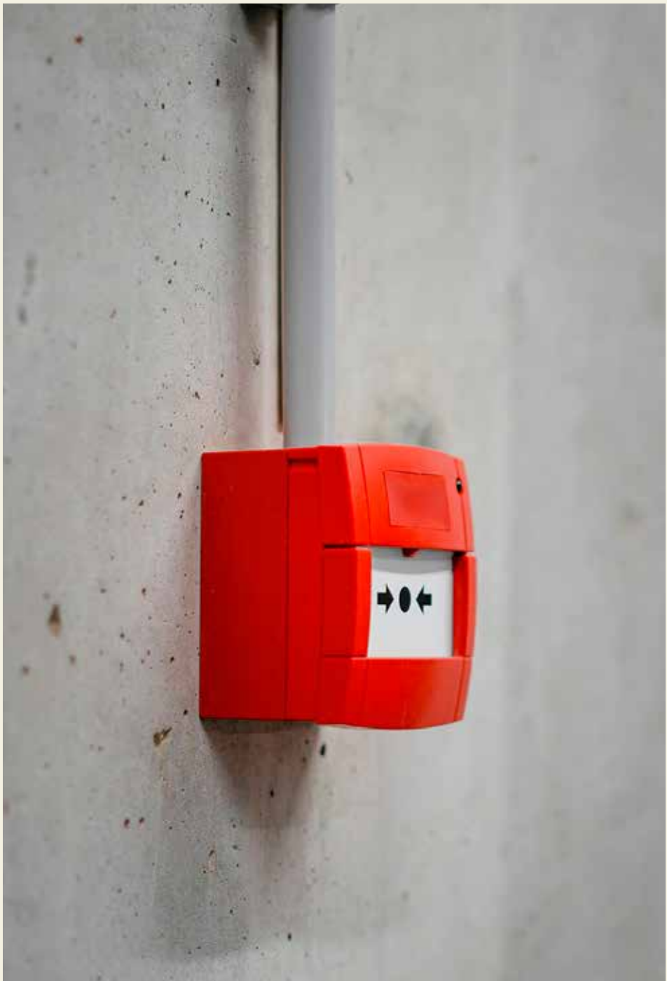
Safe fire exits
